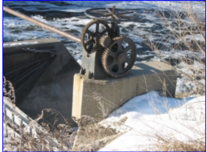
Mill Dam Gate Control
